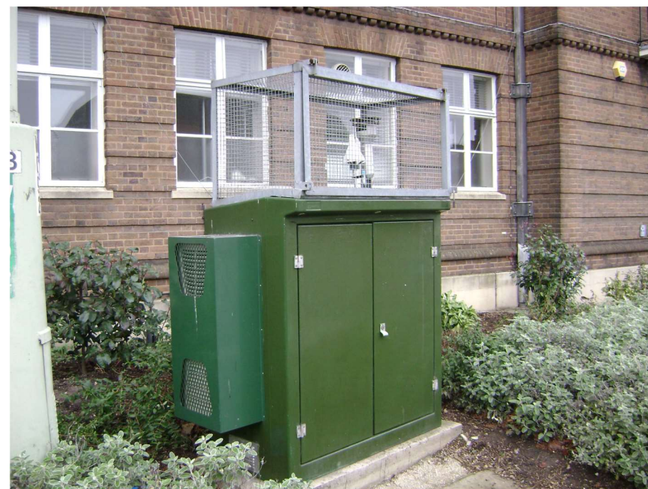
Photograph showing the automatic monitoring at Watford Town Hall.
